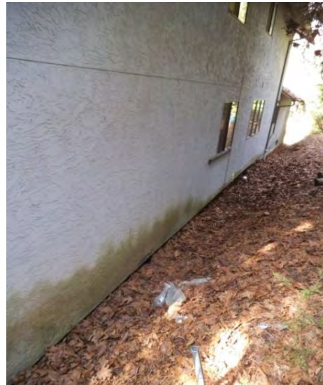
East Side of House, Surface Water Collects
