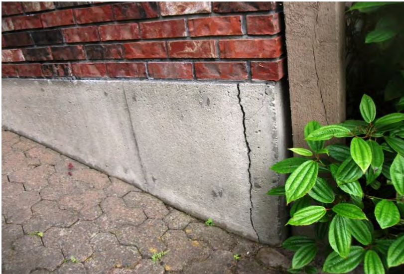
Crack In North Side Foundation
