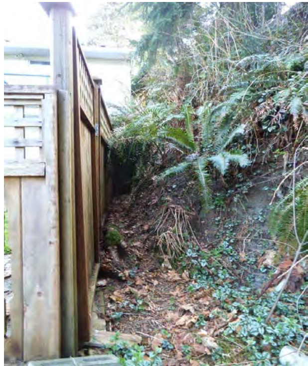
Steep Unsupported Soil Face Southwest Corner of Yard
