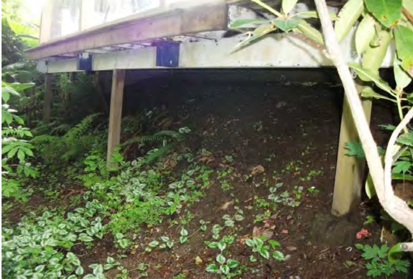
Crest Under Wooden Patio
