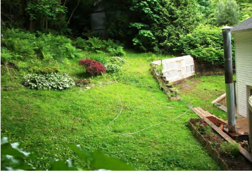
Wet Part of Timber Retaining Wall
