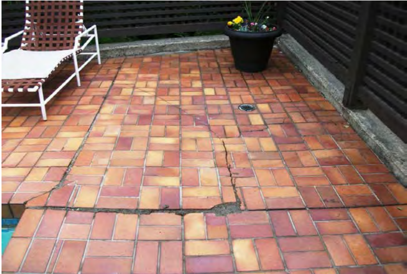
Pool With Repaired Cracks
