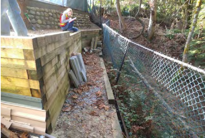
South Edge of Swale Below Crest With Damaged Maple Trees
