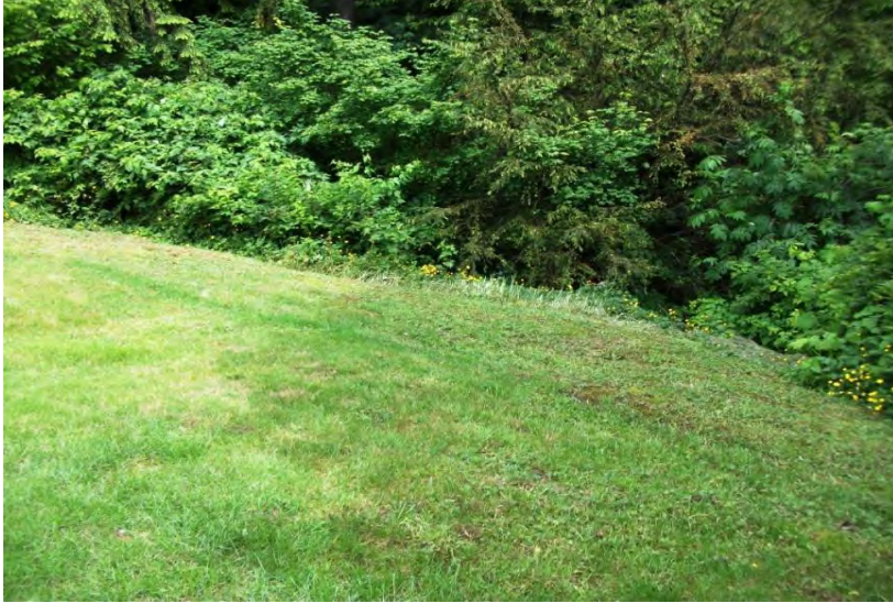
View Of Fill Apron At Crest Of Ravine With Subsidence
