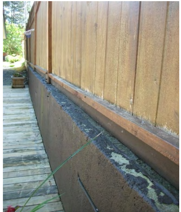
Concrete wall on north side of property, no cracks or alignment issues.
