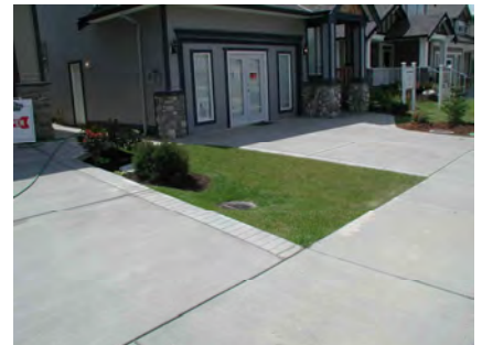
Completed single family lot infiltration trench completed; lawn basin is the only visible indication that it is there.
