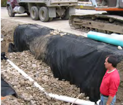
Perforated pipe over drain rock reservoir at infiltration trench under construction in Maple Ridge.
