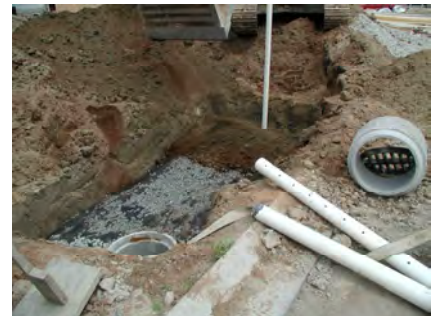
Single family lot infiltration trench being installed in East Clayton development, Surrey, BC.
