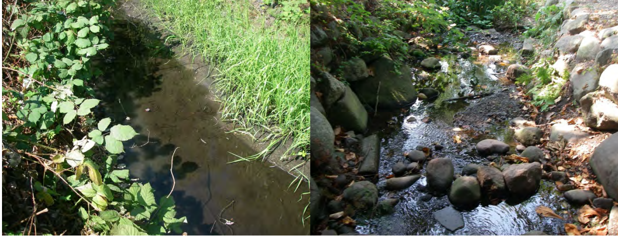
Nelson Tributary prior to realignment, with extensive invasive plant growth on the banks, summer 2010
