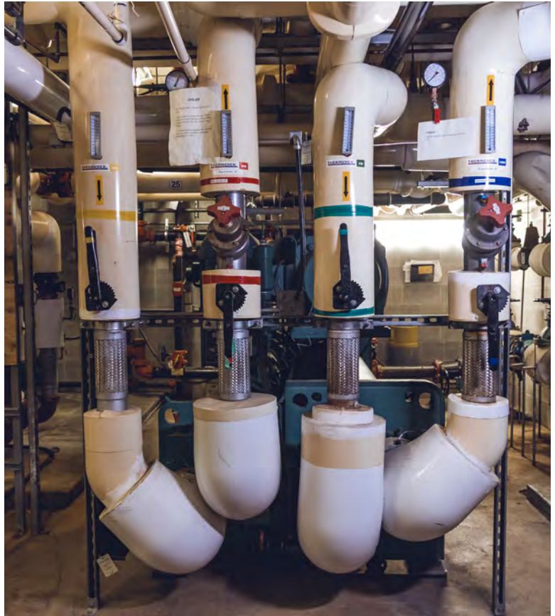
Thermenex system at Poirier Sport and Leisure Complex. This low carbon, high-performance HVAC system reuses heat and energy on-site resulting in significant reduction in energy cost and carbon emissions.
