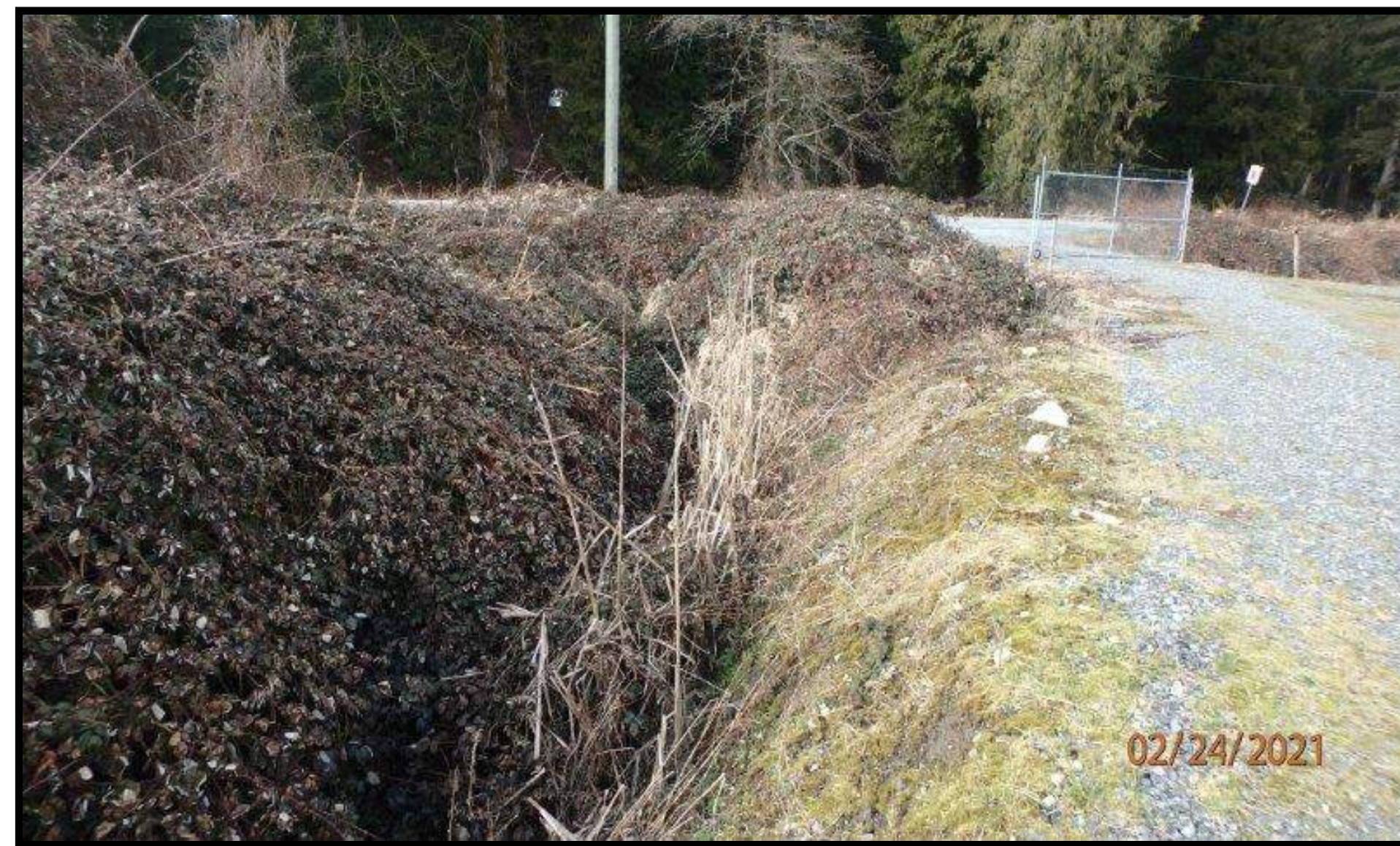
Figure 4. Upstream view of Ditch 1. Note lack of functional riparian habitat.
