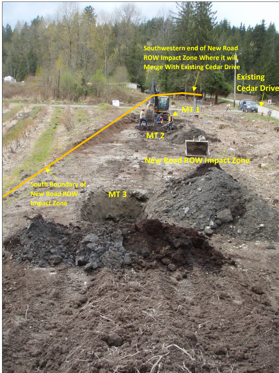
Figure 20. Location of machine tests (MT) 1 to 3 placed within area lying west of the proposed pumping station at the very southwestern end of the proposed new road bed construction at 4170 Cedar Drive, looking west from beside the proposed pumping station location towards the proposed merger of Cedar Drive and the new road ROW. Deep machine testing revealed an abandoned hard-packed farm access road bed lying on top of a very thick deposit of imported fill that rests on a deeply buried deposit of waterlogged peat and other organics consistent with a marshy/boggy environment (dark matrices). Archaeological site potential is considered to be low in this location, as it would have been a marshy/boggy low-land prior to being capped with imported fill. This section of new road ROW will be capped with sand/gravel road-base fill in mid-2022.
