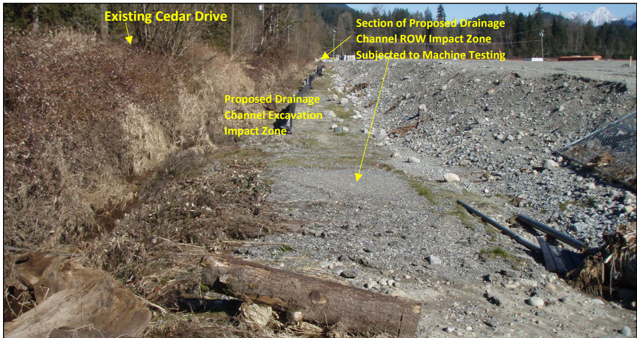
Figure 27. A February 22, 2022, general view of the west side of the north-central section new road ROW (upper right) in Development Area 7 showing section of new road-bed capped with pre-load fill in 2021 (right), looking northeast. This section will be capped with an additional 1.0 m of road-base fill in mid- to late 2022. A new drainage channel will be dug between existing Cedar Drive (upper left) and the new ROW. The area immediately west (left) of the road-bed in the center of the photo was subjected to machine testing (MTs 4 to 14) (Figures 24 and 25; Appendices III and IV).
