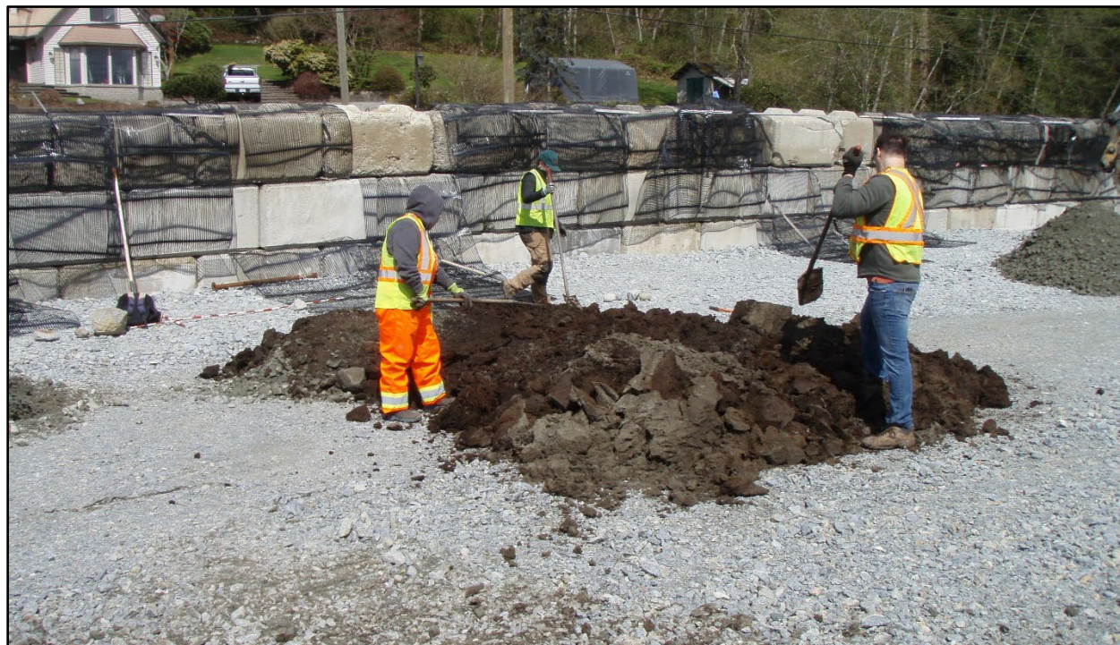
Figure 33. A view of hand-raking and close inspection of sub-fill “natural” silt and peat sediments removed from machine test (MT) 16 in progress within the new road ROW that was capped in 2021, looking north.
