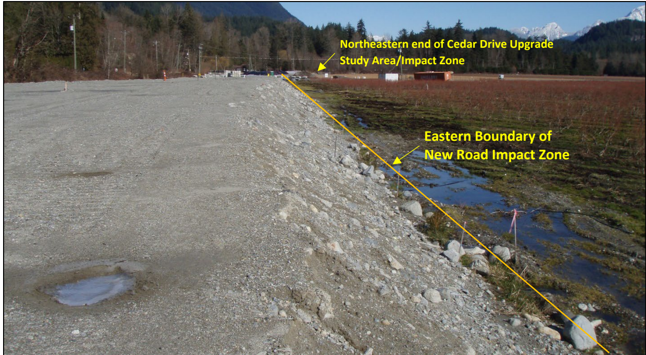
Figure 26. A February 22, 2022 general view of the east side of the northern 2/3 of new road ROW in Development Area 7 showing road-bed that was capped with sand/gravel road-bed pre-load fill in 2021, looking northeast. This section will be capped with an additional 1.0 m of road-base fill in mid-2022. Note standing water in saturated natural and imported fill deposits in lower right that indicate a high water table.
