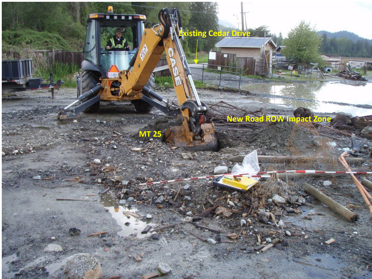
Figure 23. Excavation of MT 25 underway within the proposed new road ROW about 20 m east of the proposed sanitary force main pump station within the southwestern aspect of 4169 Cedar Drive, looking northeast. It is proposed that this area will be capped with road-base fill in mid-2022.
