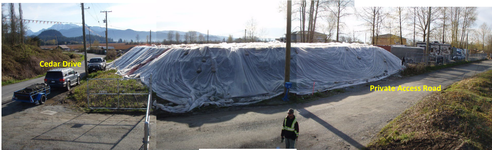
Figure 9. A panoramic view of the large pile of sand and gravel preload that currently occupies the location selected for the sanitary force main pump station (Development Area 5) at 4180 Cedar Drive, looking southeast. The sand and gravel preload will be removed in June, 2022 and transported to Development Area 7 (see below) where it will be placed on top of existing similar preload deposits within the new road ROW.
