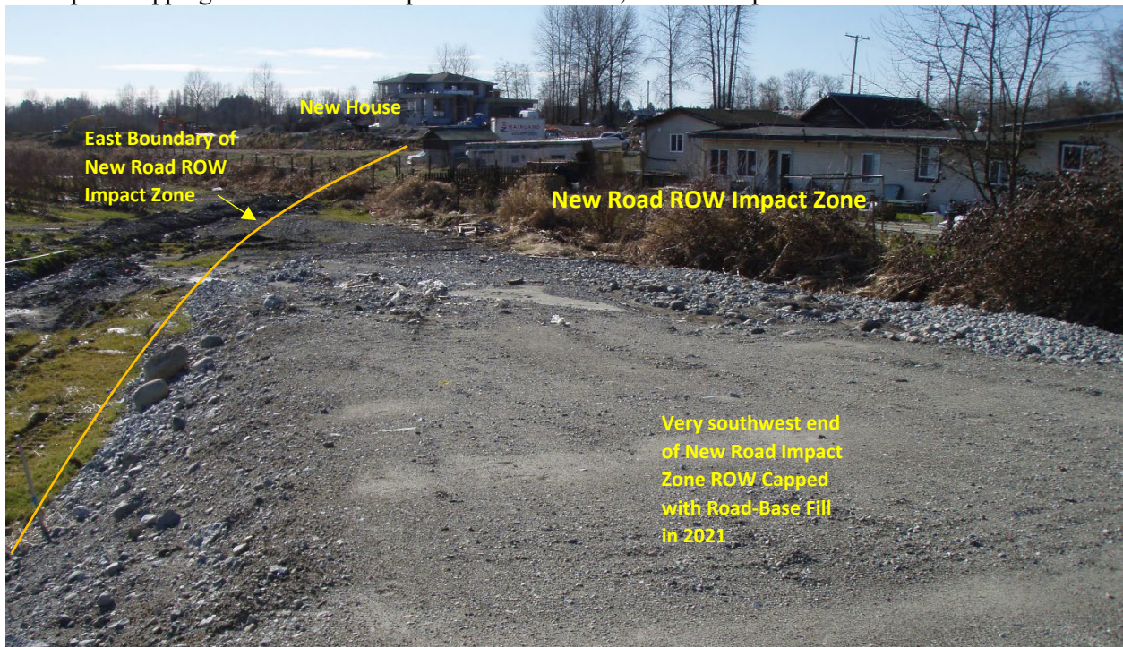
Figure 19. A view of the north end of the yard/pasture at 4169 Cedar Drive within the new road ROW (upper right), looking southwest from the very southwest end of the road-base fill (foreground). This area will be capped with road-base in mid-2022 after the buildings etc. are removed.
